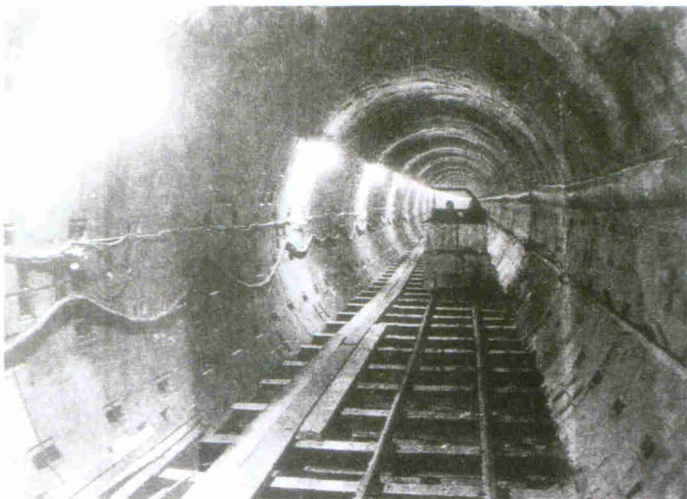
合流污水一期工程 The First Stage of Combined Sewage Projection
